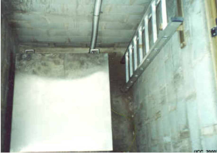
Detail of the steel box at the bottom of the seismic vault.
