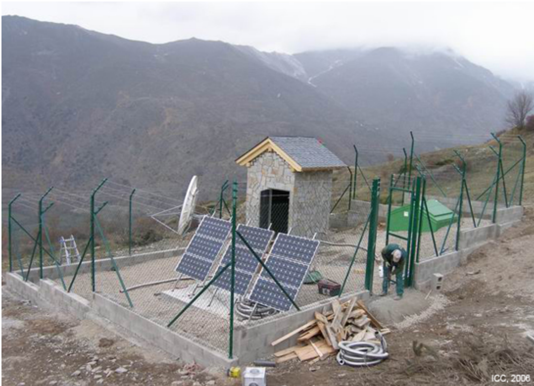
General view: VSAT antenna, instrumental house, seismic vault cover, solar pannels solars and fence.
