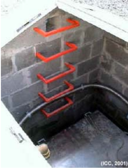
Views in detail of the cover of the seismometer vault and staircase of access to the steel box where it meet the sensor.
