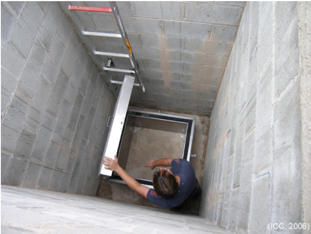
Seismometer vault at 3 m of depth
