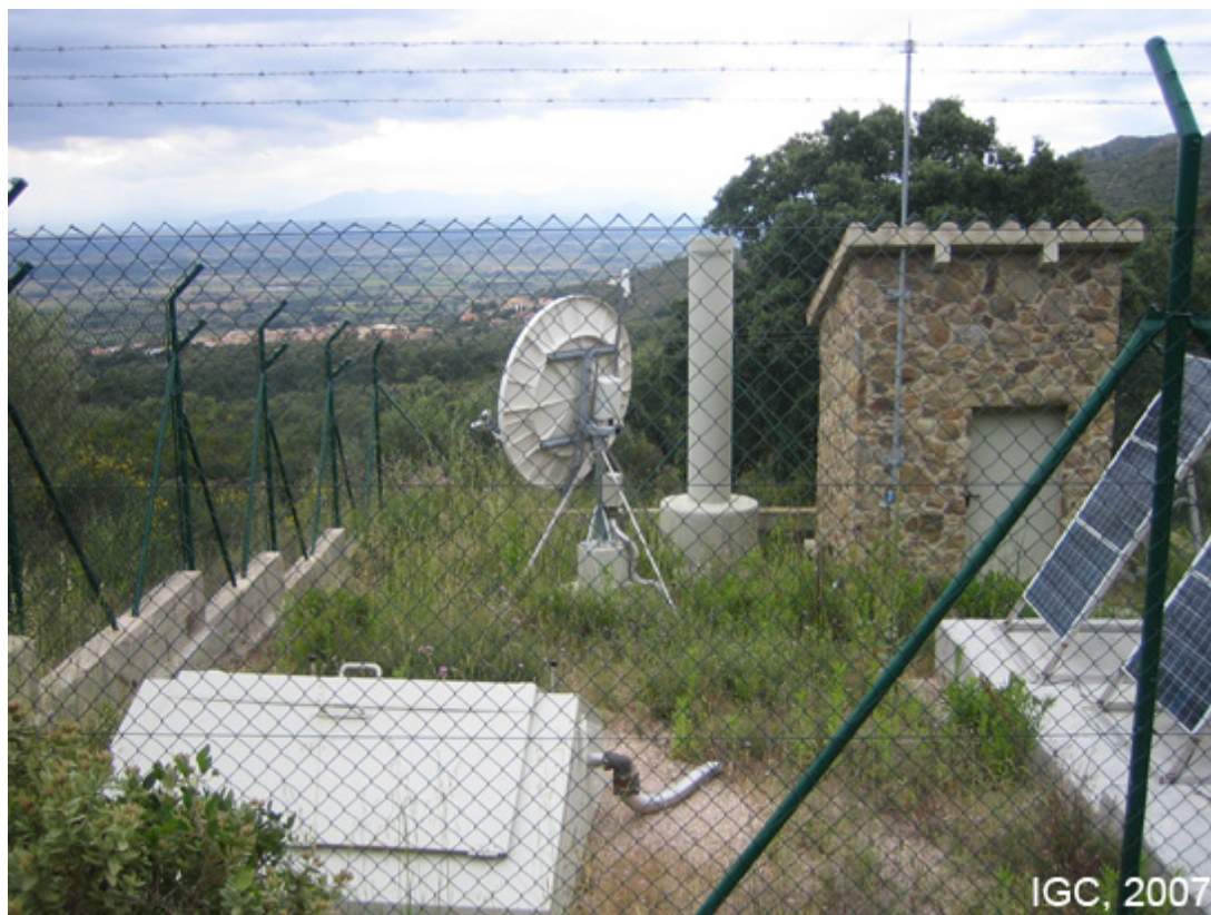
General view: seismic vault cover, solar pannels, instrumental house, geodetic pillar, lightning rod, VSAT antenna and fence.
