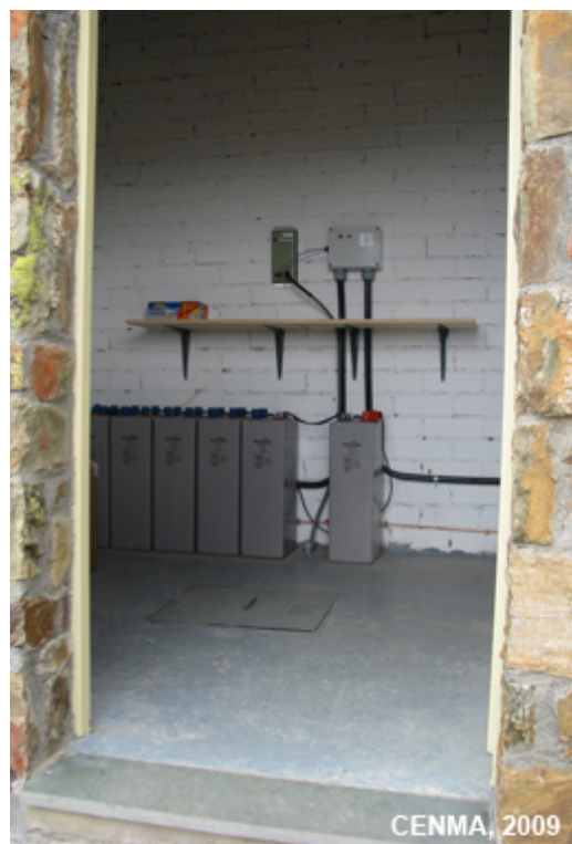
Instrumental house: Detail from inside the instrumental house with the feed system batteries and access cover in depth sensor
