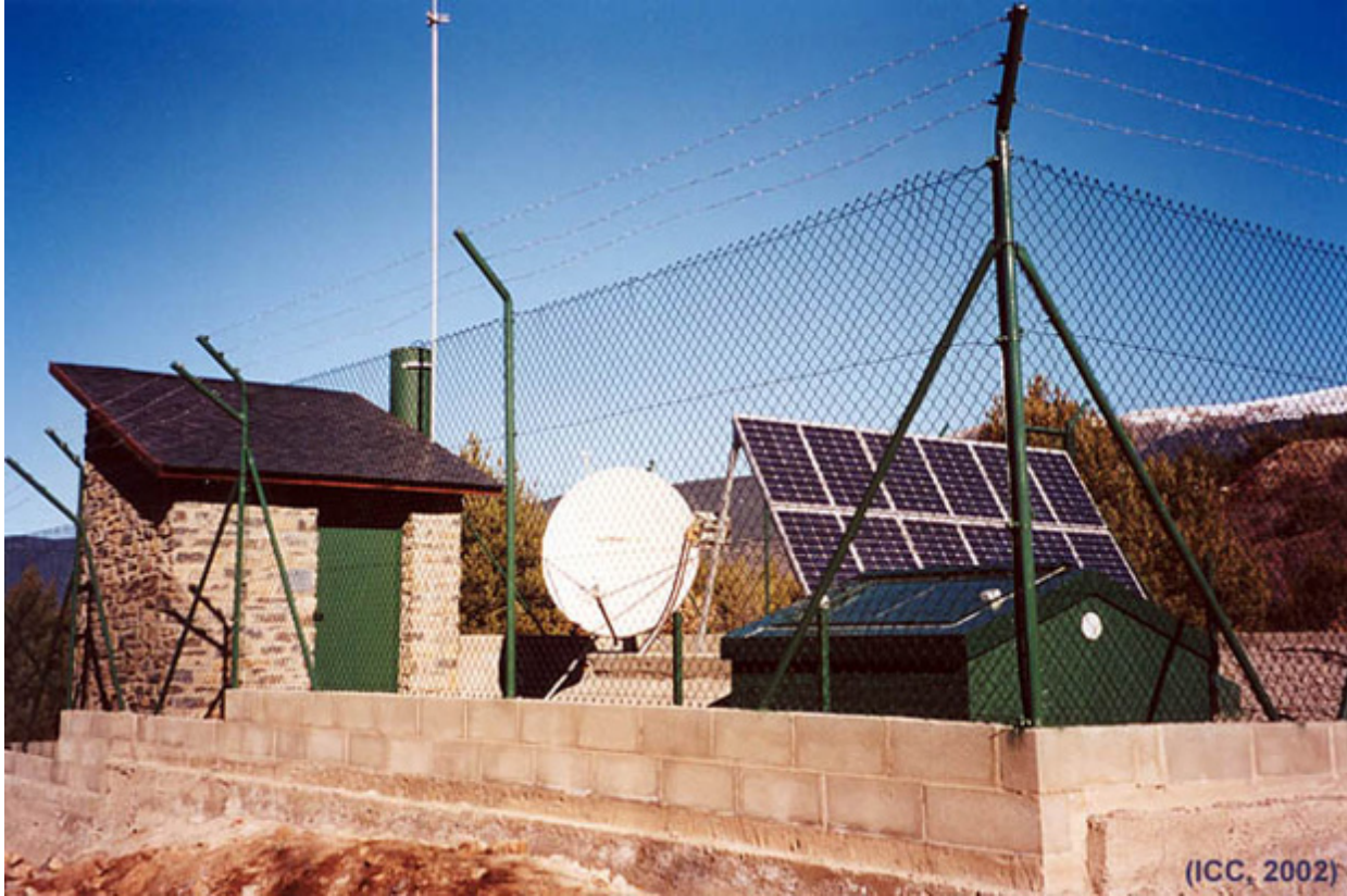
Lateral view of the Soriguera seismic station. You can observe the lightning rod (PDC) just at the right side of the geodetic pillar.
