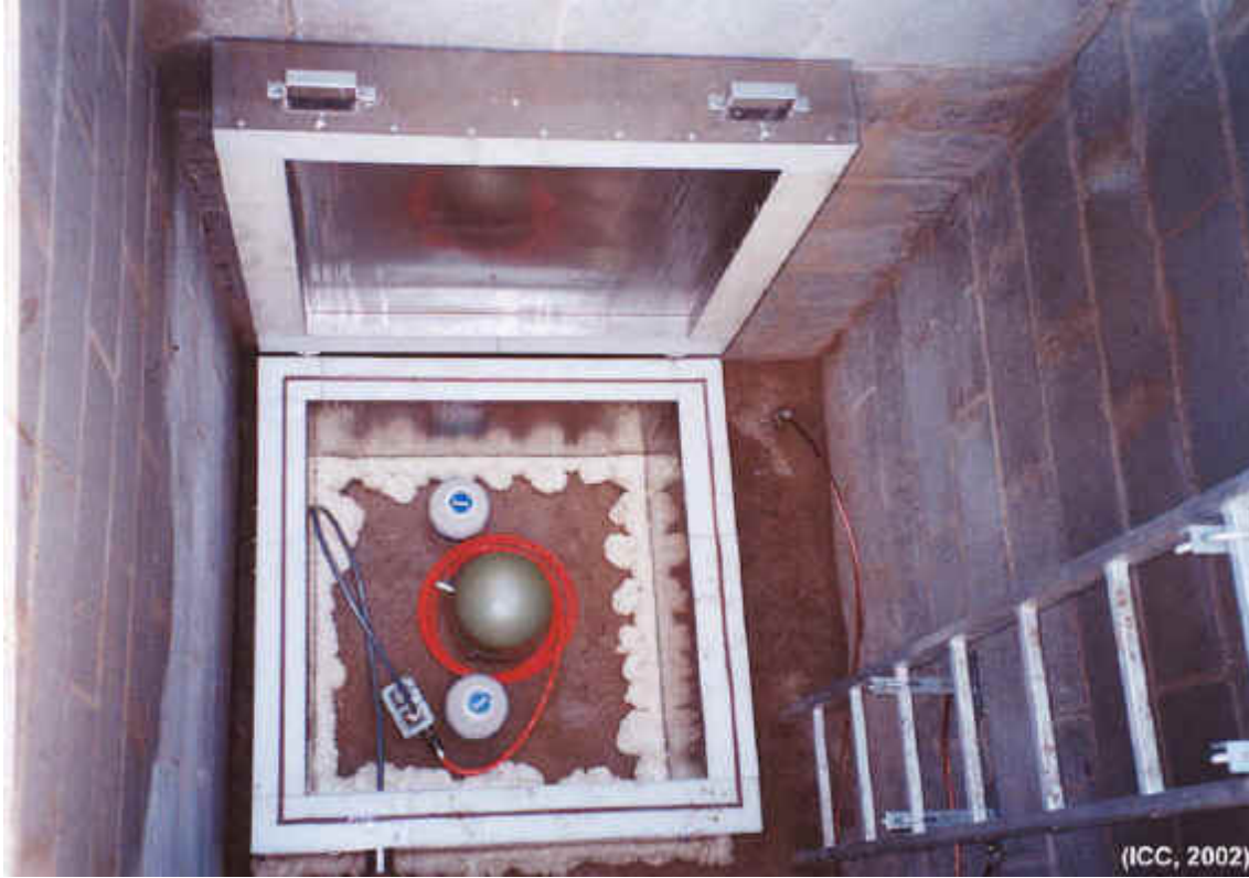
View in detail of the seismometer vault and the staircase of access to the steel box where it meet the seismic sensor.
